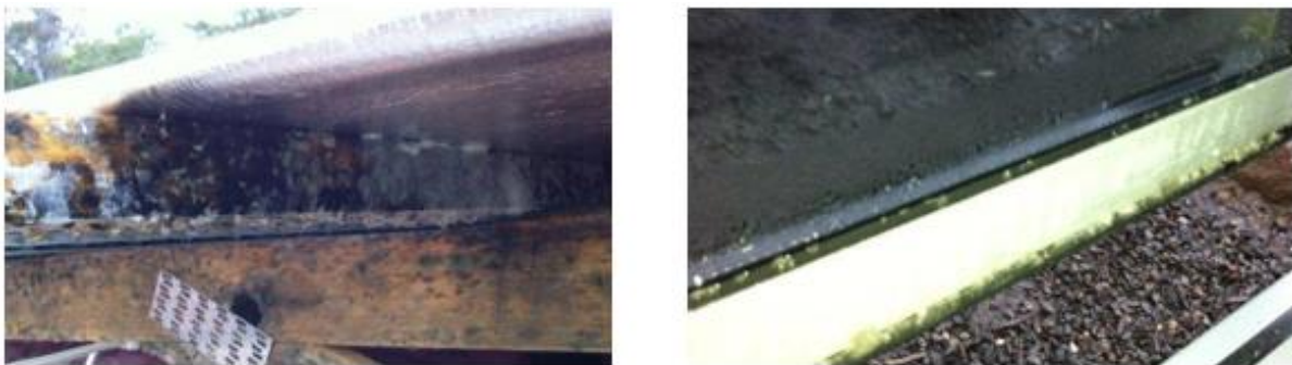
Figure 15 – Condensation and mould inside roof space and condensation and mould on double glazed window and aluminium frame
