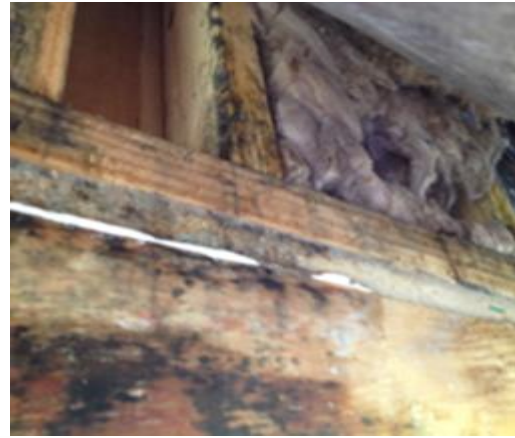
Figure 9 – Wet wall insulation, wet timber structure and mould growth within wall
