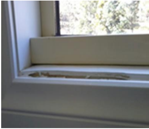
Figure 6 – Expanding timber elements resulting from excessive moisture in the built fabric
