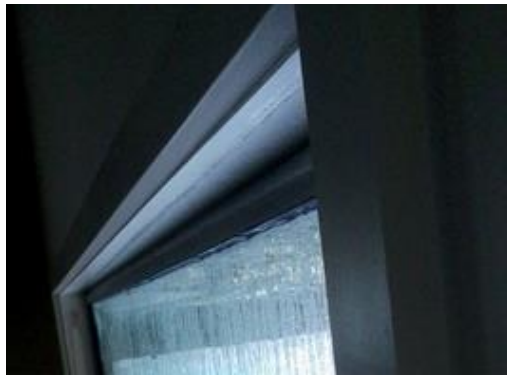
Figure 7 – 'Raining' windows resulting from excessive moisture in the built fabric
