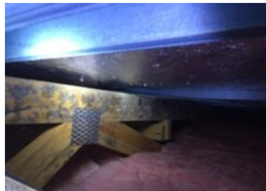
Figure 11 – Mould growth in overly moist roof space
