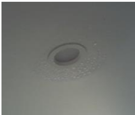
Figure 8 – Moisture forming around ventilated and uninsulated downlight
